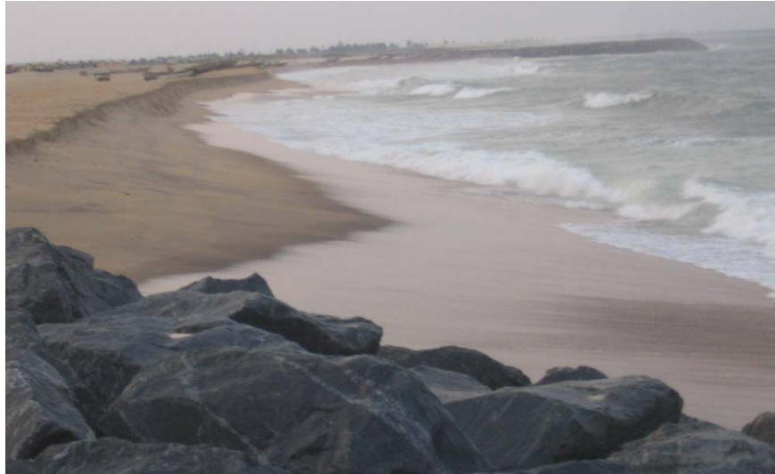
Plate 2 Erosion between Defence Groynes at Keta
