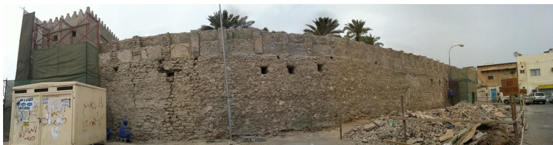
Fig 5.2 Sheikh Salman house as it exists now in dilapidated condition.
