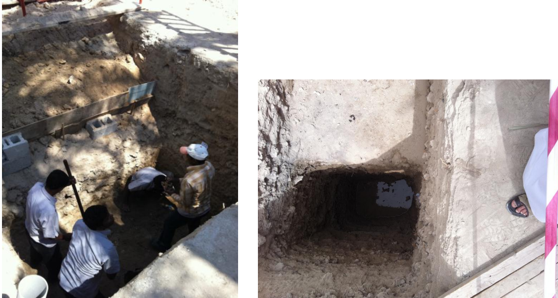
Fig 5.1. Excavation at Sheikh Salman house, showing the ground water at around 4.5 meter depth.
