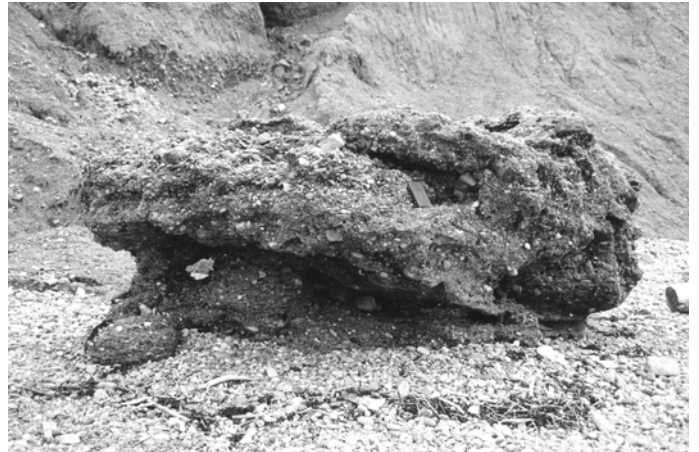
Figure 7. Fallen block of the indurated cobble gravel unit, indicative of a possible rockfall hazard below the cliffs.
