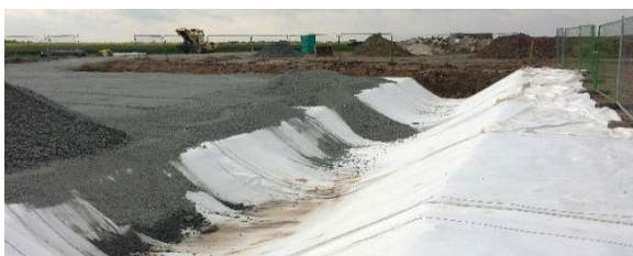
Figure 7: Geotextile wrapped shear trench under construction, before being wrapped back under platform.
